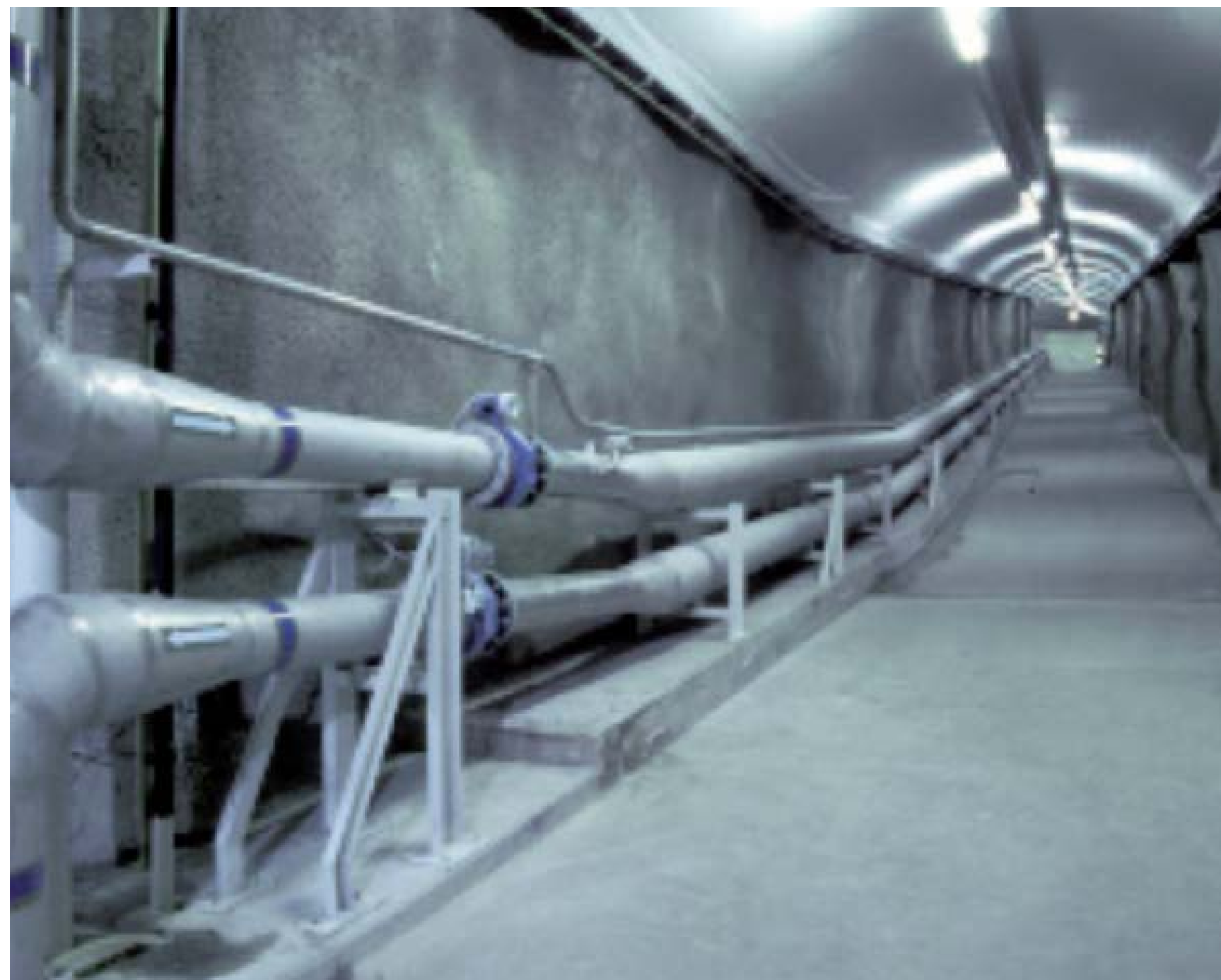
Detail of the drinking water treatment plant at Lake Como, Italy. Picture courtesy of Centro Inox.
