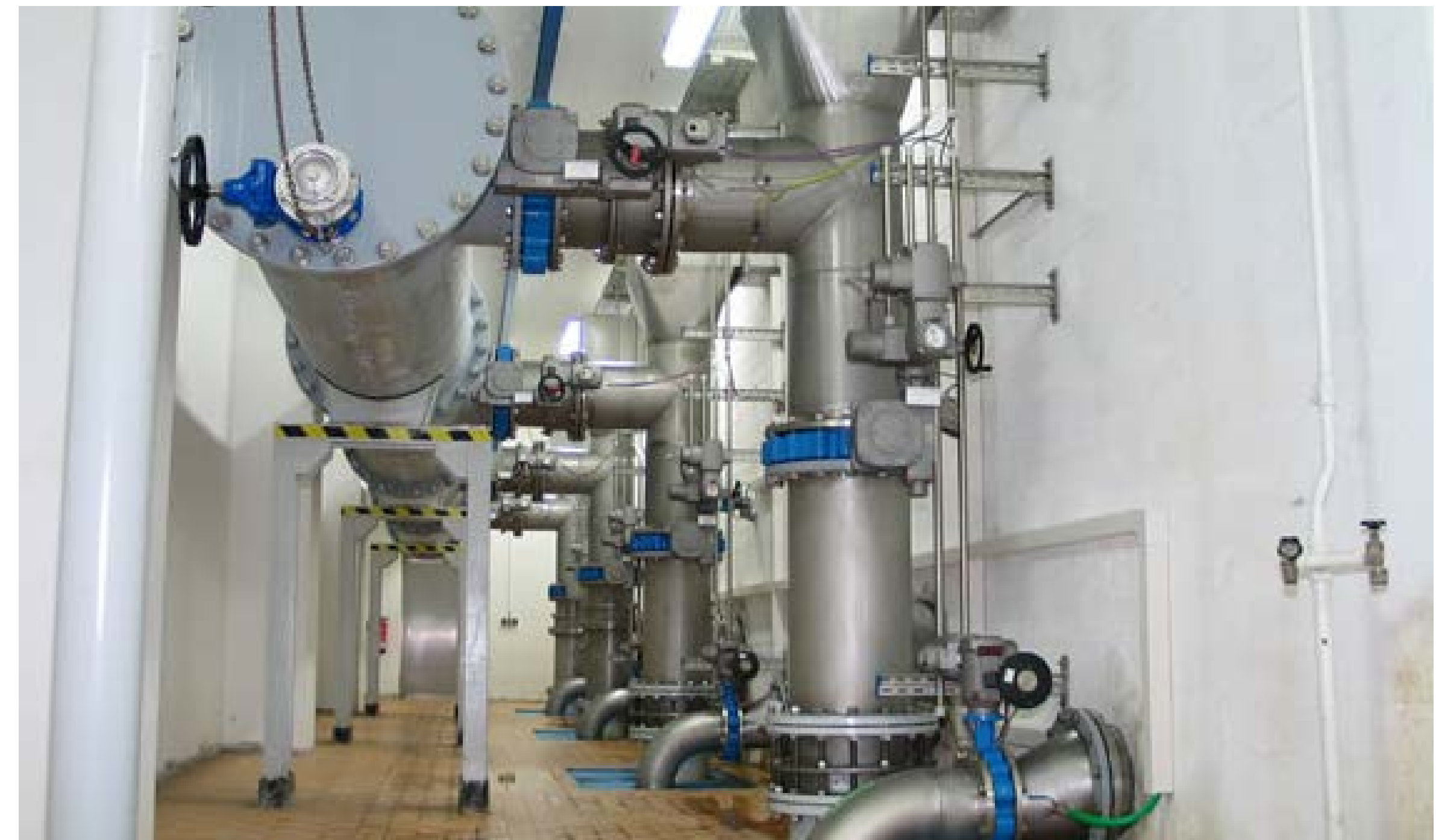
Stainless steel in municipal waterworks. Picture courtesy of Schenke Anlagenbau
